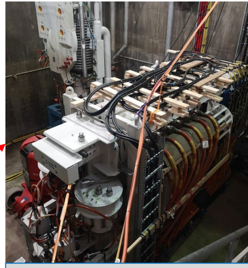
Subsea Step-down transformer in test pit
